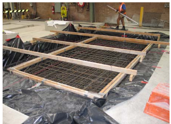
The isolated plinth before paving (the plinth supports the vibrating machinery)
