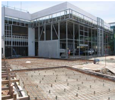
Steel to paving inspection Late November 2004 - 3 days later how quickly things change
