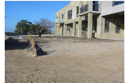
Some of the more than 700m 2 of concrete paving being reinforced during the final stages
