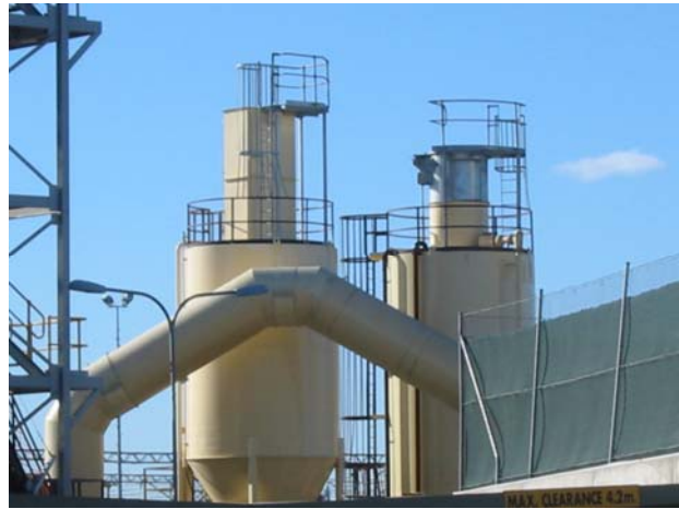
After: Safety rails, platforms and ladders were installed for maintenance access to the very top of the silos.
