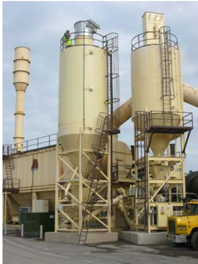
Before: This photograph was taken of the silos on our initial inspection.
