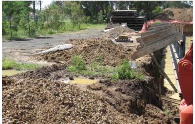
The shutters on the far right are on the boundary. No permission had been obtained for these walls by the neighbours.
