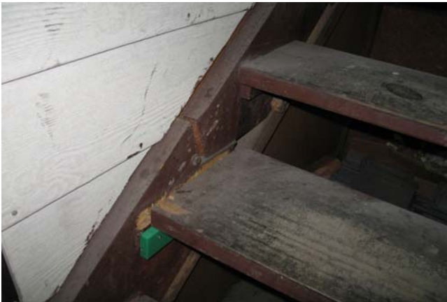
This side of the stairs was bad
