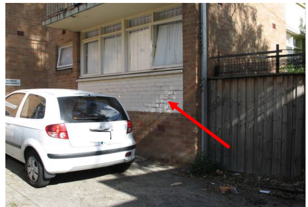
Shows the crack in the wall
