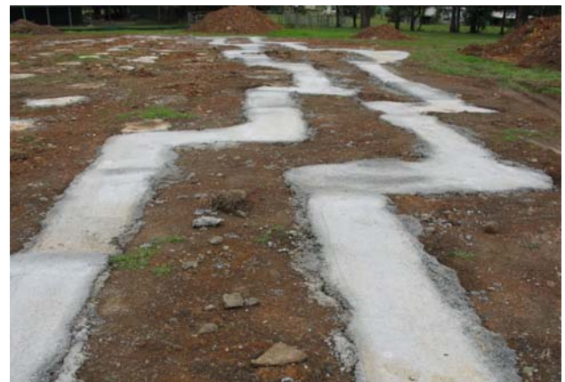
Some of the many footings to be repaired
