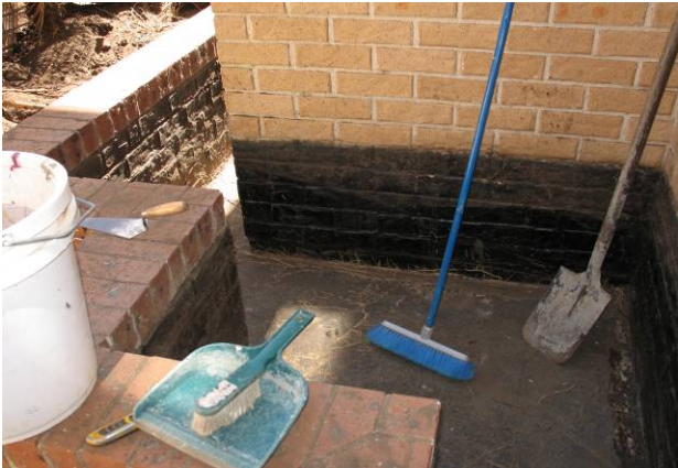
Roots had penetrated existing waterproof membrane.
